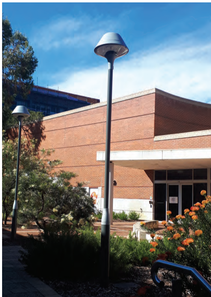
Image 13. Image shows existing Curtin light poles which are to be utilised for the Circuit.
